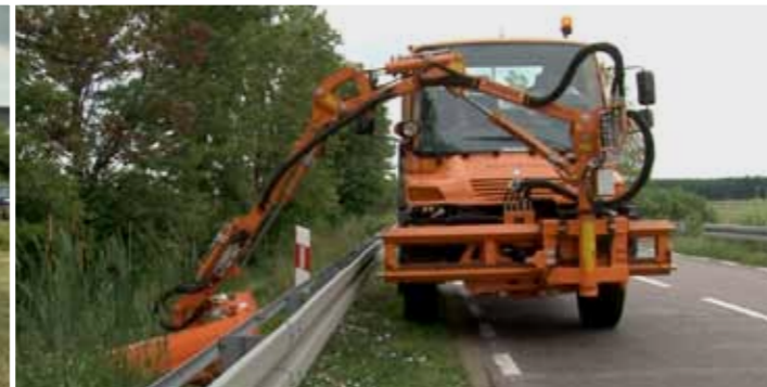
Mowing of a hard-to-reach roadside using a WWP500U multifunction arm and GK 110 head.
